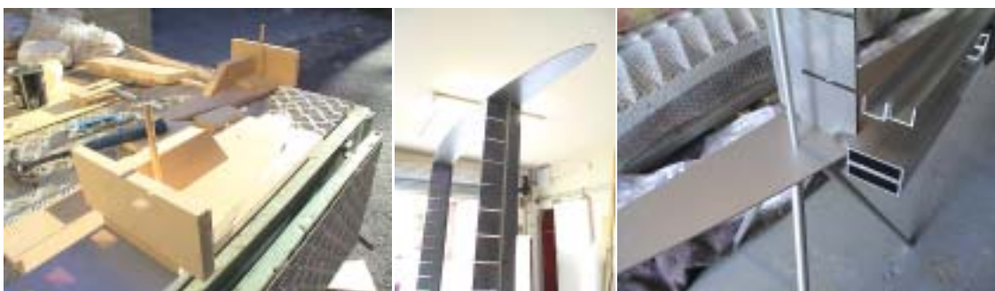
Above: Detail of the welding jig for the acrylic partition screen chassis, detail of the welded chassis, detail of the stiffening beams prior to installation
