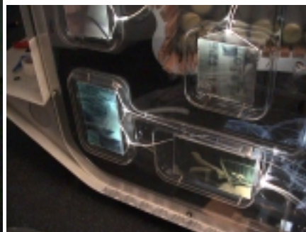
Left and above: Images of the first fibre optic loom and light guide installation into Screen Lounge pod 01. The uncoated optical fibres are visible through the
